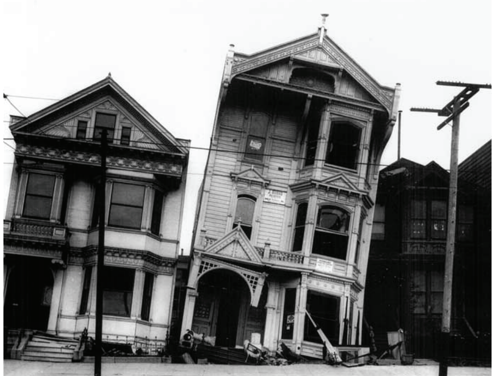
San Francisco homes damaged in the 1906 earthquake. Photo credit: Courtesy of the National Information Service for Earthquake Engineering, University of California, Berkeley.
