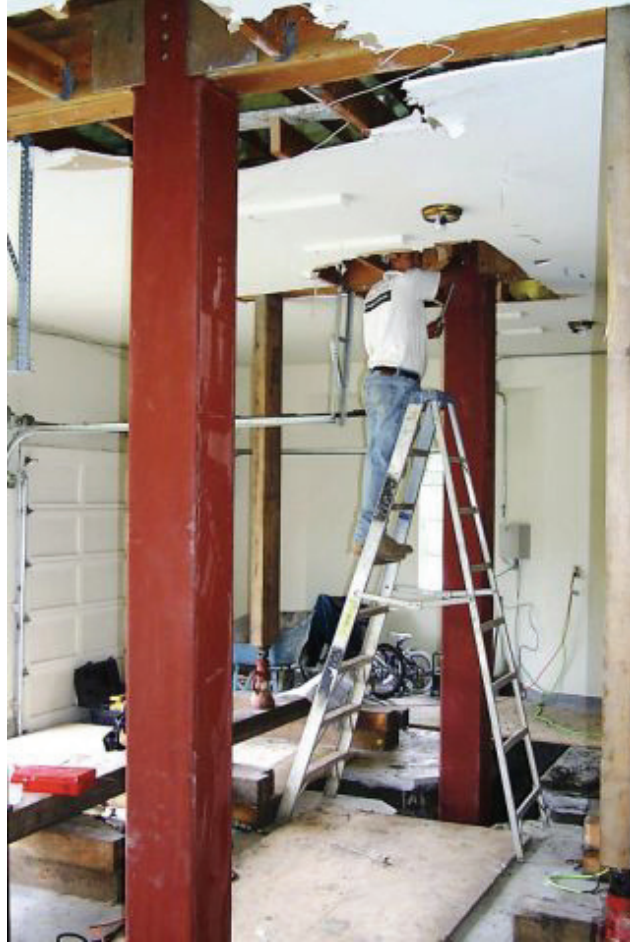
A seismic retrofit in progress. Photo credit: Courtesy of Anderson Niswander Construction.
