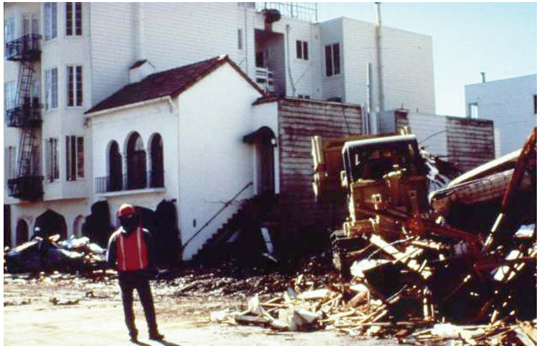
Demolition in the Marina District after the 1989 Loma Prieta earthquake. Photo credit: Courtesy of Earthquake Engineering Research Institute Mitigation Center, Oakland, California.
