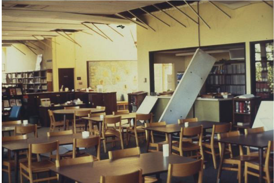
: A heavy ceiling panel that fell in a private school in the 1987 Whittier Narrows earthquake in southern California. Photo credit: Earthquake Engineering Research Institute Mitigation Center, Oakland, California.
