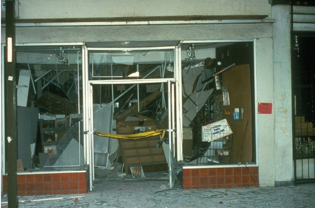
A store damaged in the 1989 Loma Prieta earthquake with damage that will delay occupancy. Photo credit: James Blacklock, Courtesy of the National Information Service for Earthquake Engineering, University of California, Berkeley.
