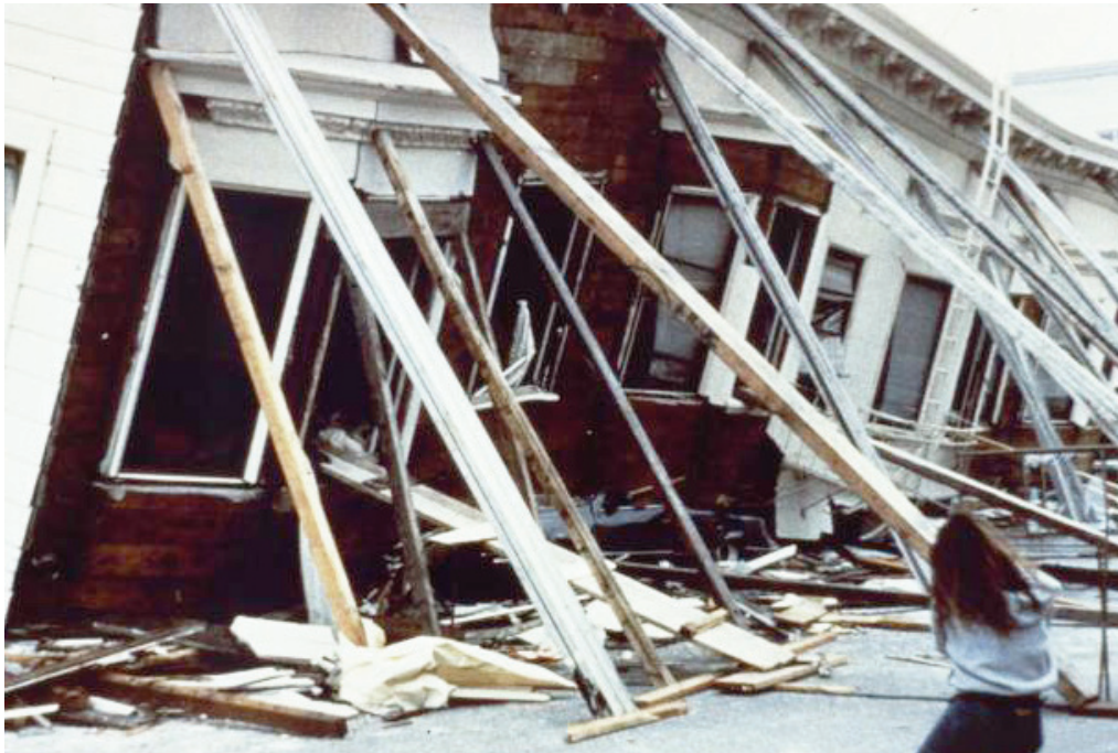
A damaged building in the Marina District after the 1989 Loma Prieta earthquake. Photo credit: Courtesy of Earthquake Engineering Research Institute Mitigation Center, Oakland, California..
