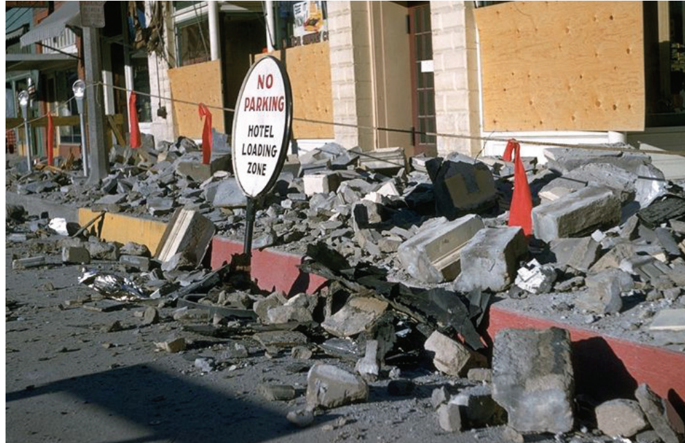
Damage to a Hotel in Nevada after an earthquake. Photo credit: Karl Steinbrugge, Courtesy of the National Information Service for Earthquake Engineering, University of California, Berkeley.
