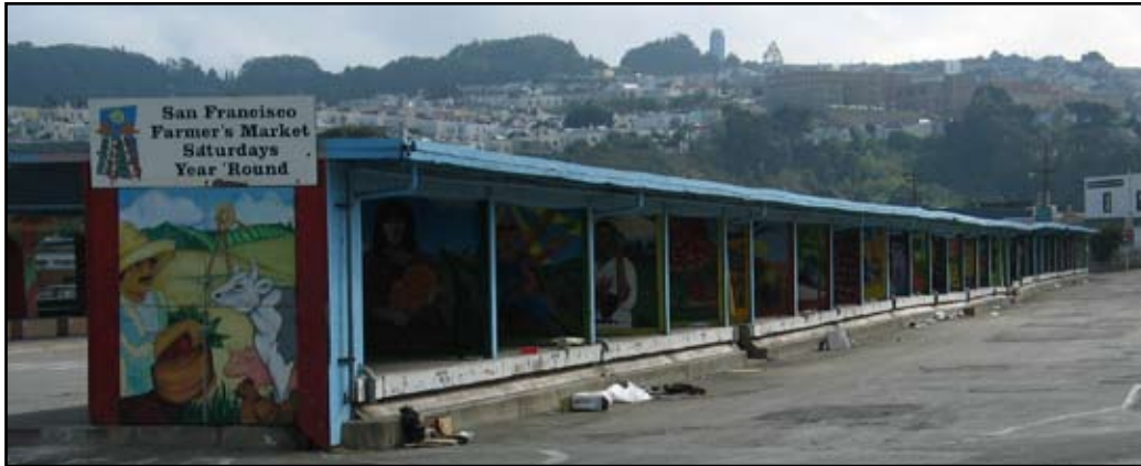
The roof at Alemany Market, one of several facilities the General Services Agency maintains, is being repaired with funding appropriated in FY 2008-2009.
